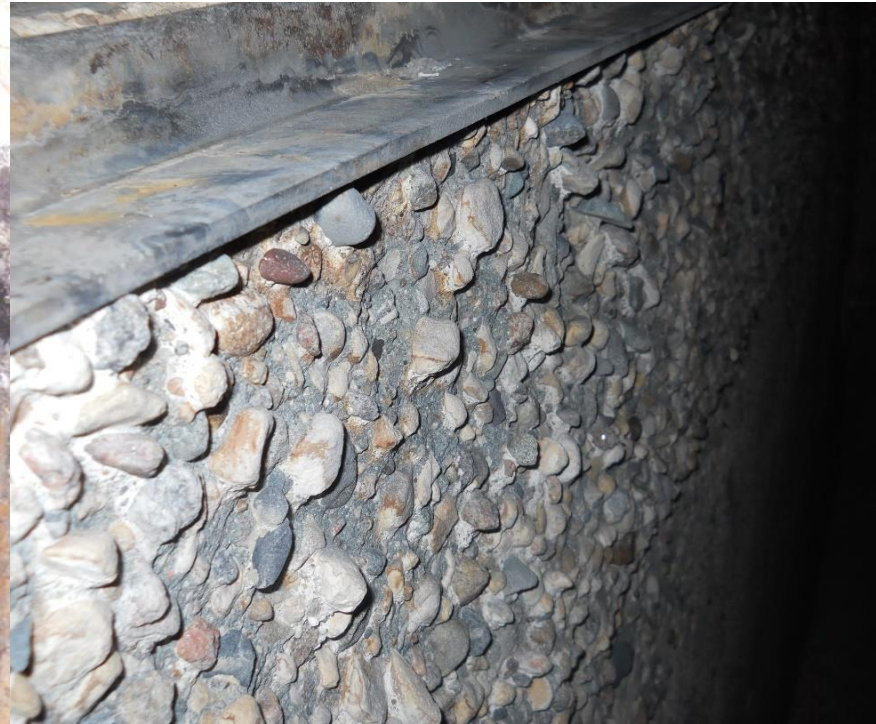
Concrete coated ductile iron pipe corrosion at the Bismarck WWTP, due to H 2 S
